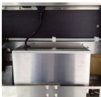
The hand dryer in situ
