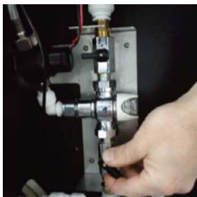
1. Isolate the water supply locally
