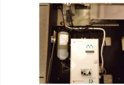
1. Locate the soap tank adjacent to the control box
