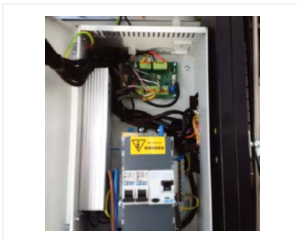
5. Control box open showing main PCB
